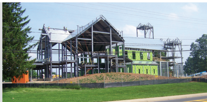
(Right) Construction of a new church for St. John the Apostle Parish, Leesburg
